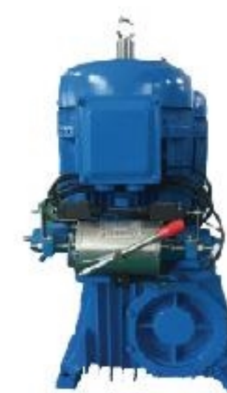
·Escalator drive main engine
