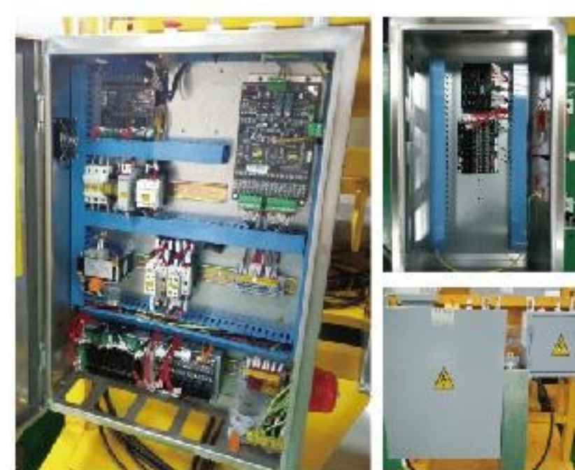
·Escalator control cabinet
